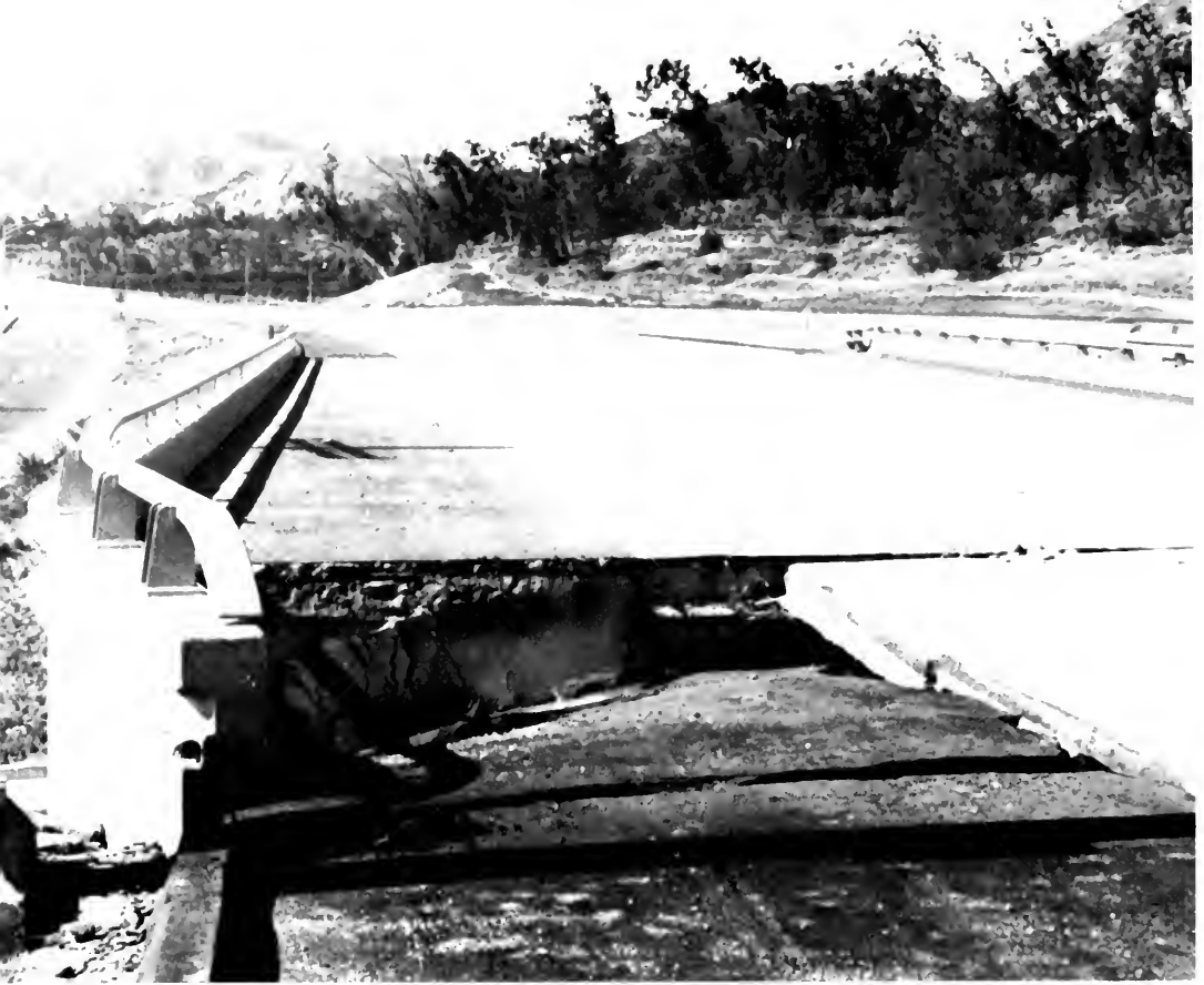
Photo 3. Settlement of bridge approach fill on Route 210.
